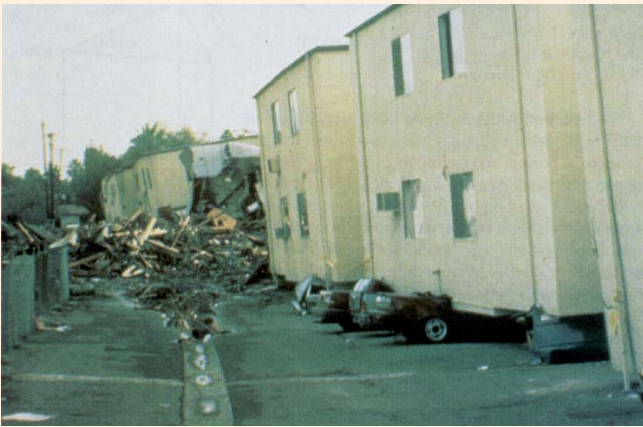
Soft-story apartment collapsed due to the Northridge earthquake
