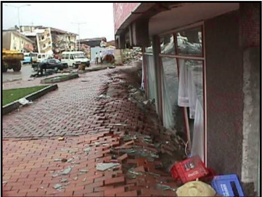
Example of liquefaction damage in the 1999 Kocaeli, Turkey Earthquake
