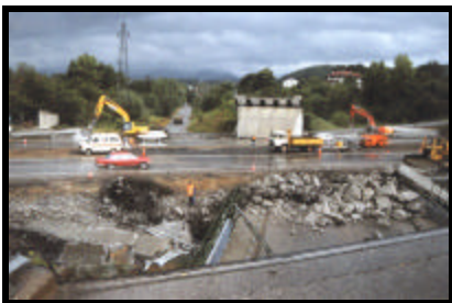
Arifiye overpass collapse following the 1999 Kocaeli, Turkey Earthquake
